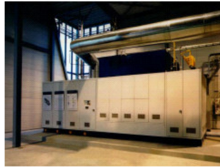
250 KW SOFC – Siemens Westinghouse
