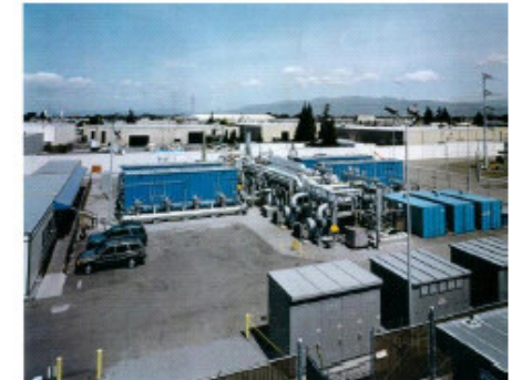
2000 KW MCFC – Fuel Cell Energy
