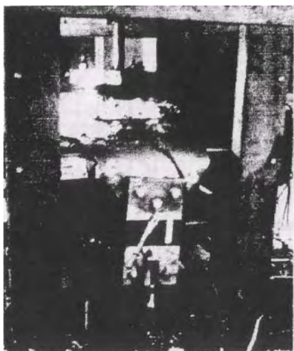
Figure 13. Homopolar generator - front view exposing the General Electric 2500 Ampere 50 millivolt current shunt.
