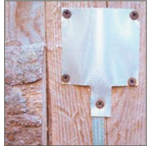
Grounded touch plate beside the entry to a gas processing area
