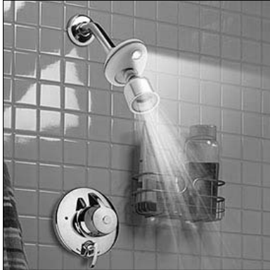
Figure 13-8: A bright approach to more efficient showering.
