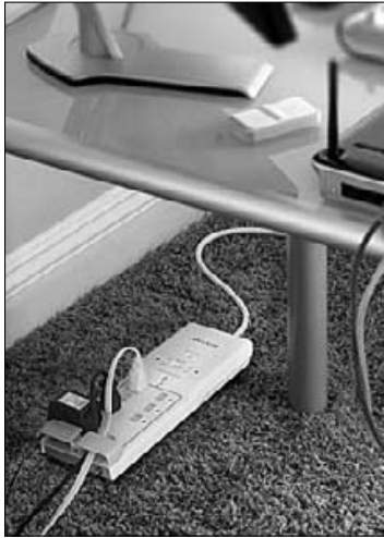
Figure 6-1: Stop sucking power from your devices by using a smart power strip.
