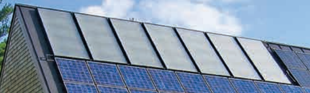
Seven Heliodyne Gobi flat-plate collectors provide domestic hot water and hydronic space heating.
