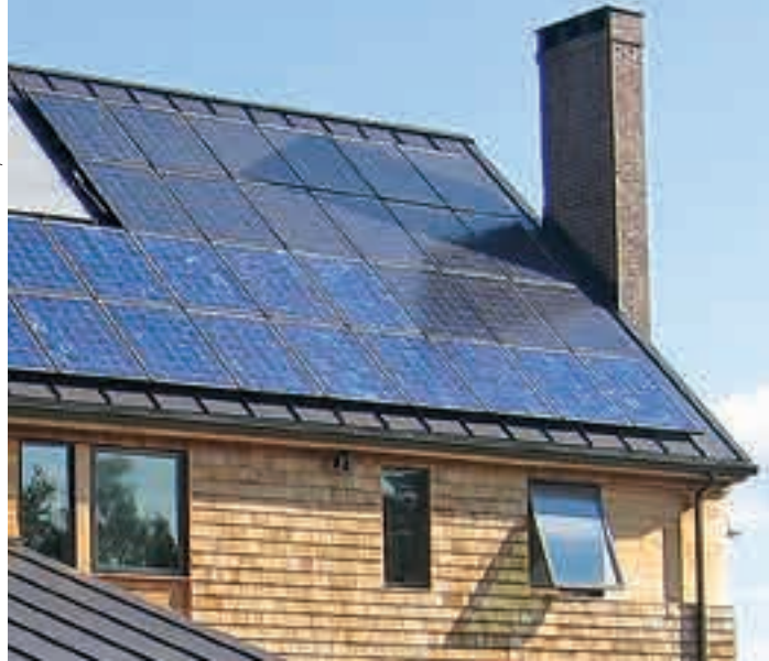
The 6.8 kW array was oversized to accommodate future loads. The array strings were configured to minimize the impact of early morning shading from the chimney.
