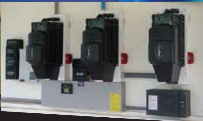
A triple stack in Hawaii using the MidNite Nottagutter
