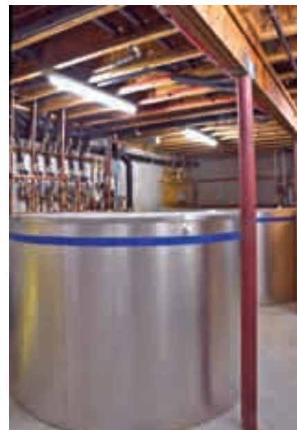
The main 738-gallon storage tank's heat exchangers serve the solar input and DHW and hydronic output loops.
