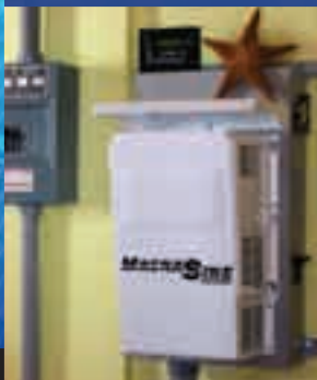
A Magnum Energy installation in Oregon
