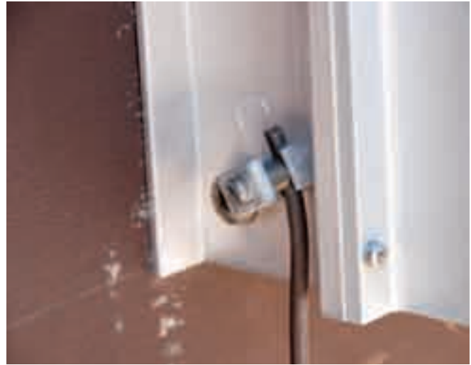
Close-up of an external grounding electrode terminal.
