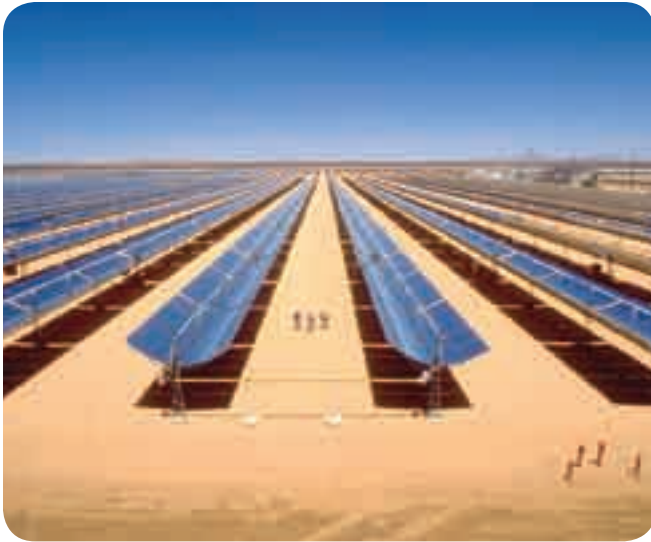
A large array of parabolic trough concentrating collectors at Kramer Junction, California.
