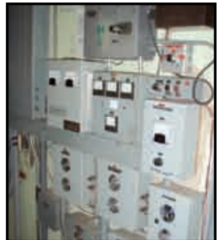
The hydro plant electrics, metering, and controls.
