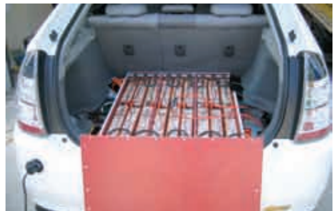
A lithium-ion battery pack in CalCars' EnergyCS/EDrive-converted plug-in Prius.
