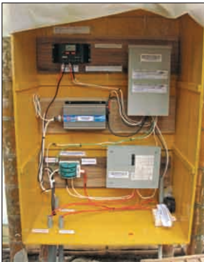
The power center, with each component labeled in Spanish and English.
