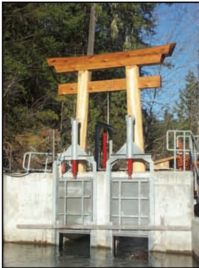
The intake gates that feed the community's hydro-electric system.
