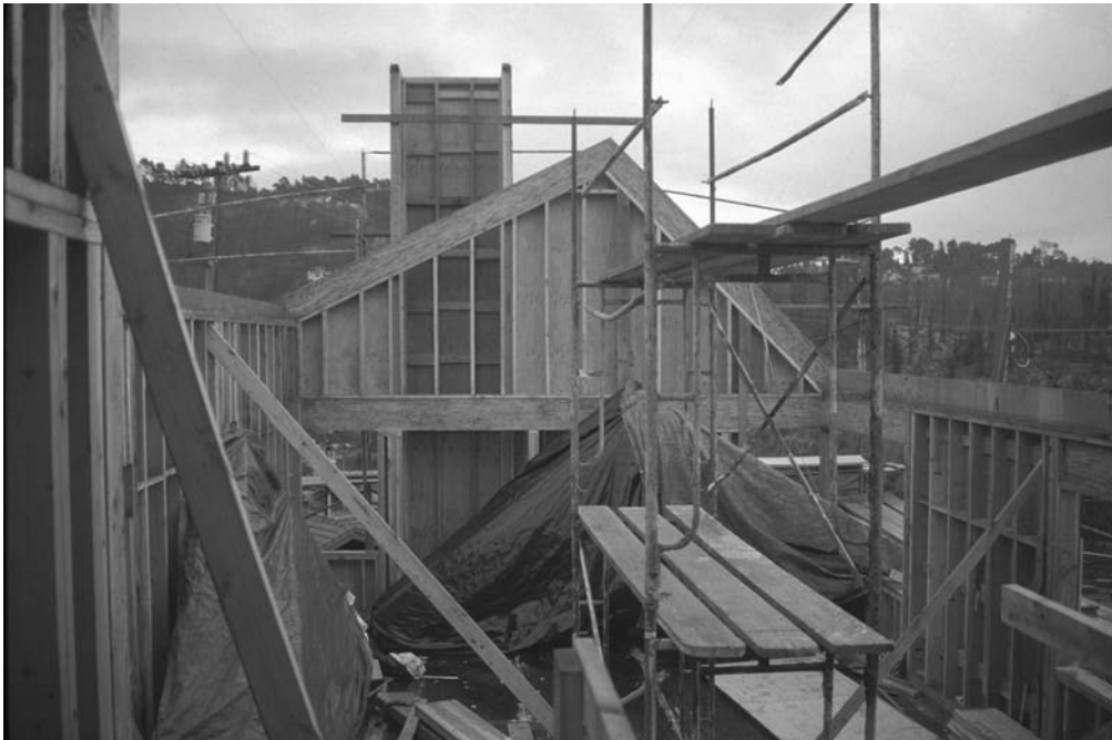
Figure A.6 Inside view of living/kitchen/dining section ready to install long rafters for solar roof.
