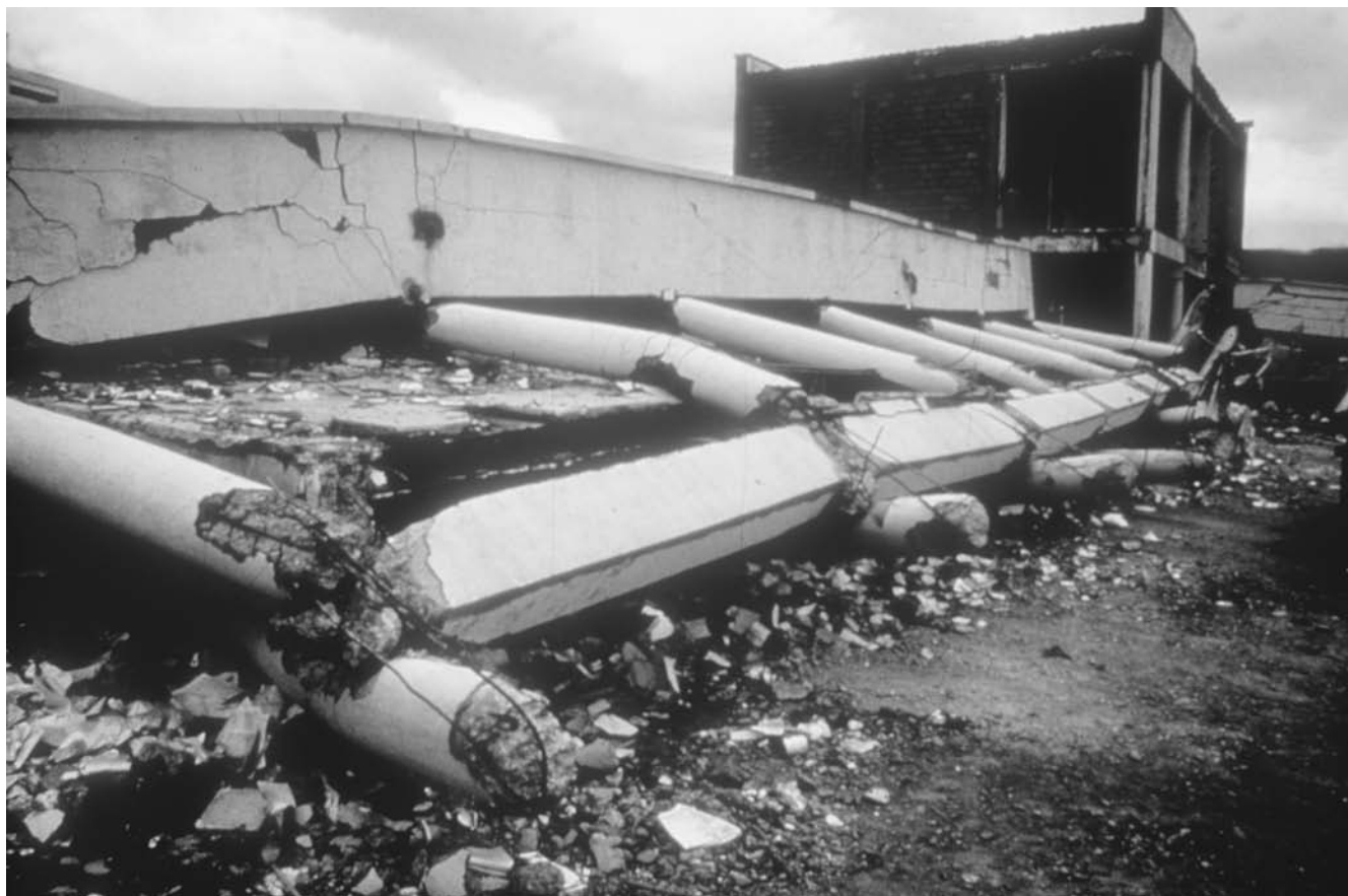
Building destroyed by surface waves from the 1980 El Asnam earthquake (Courtesy of the USGS)
