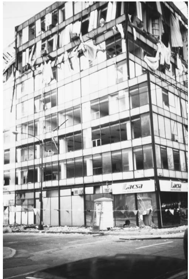
Rayleigh waves caused the crush and collapse of the upper floors of the Lasca Building during the 1985 Mexico City earthquake. Most of the windows were popped out and turned into missiles. (Courtesy of the USGS)
