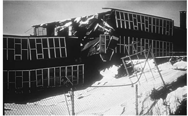
A large slump broke an elementary school in half during the Good Friday earthquake in Alaska, March 27, 1964. The earthquake had a magnitude of 9.2 and caused over $538 million in property damage. (Courtesy of NOAA)
