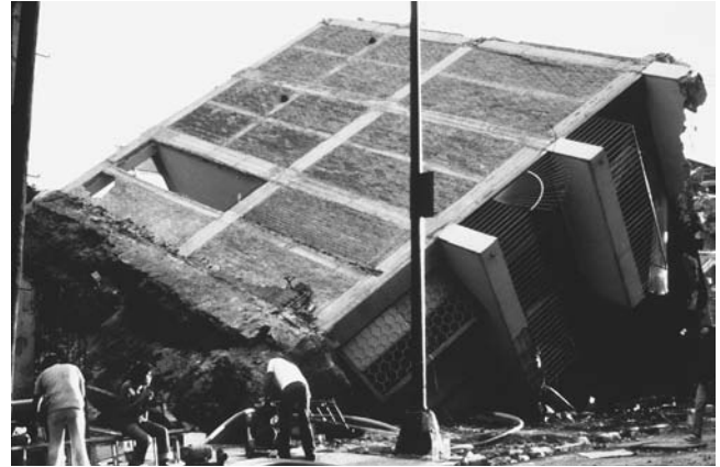
An eight-story frame structure with brick walls was broken away from its foundation and broken in half during the 1985 Mexico City earthquake. (Courtesy of the USGS)
