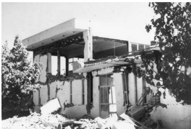
Damage to a building in Tabas, Iran, from an earthquake on September 16, 1978. (Courtesy of the USGS)
