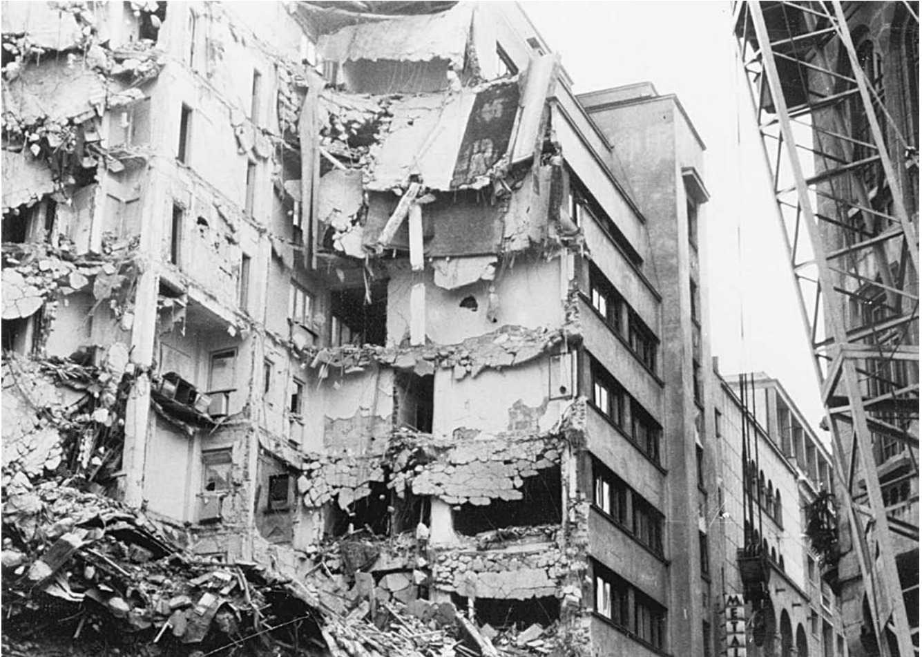
The 1977 earthquake in Bucharest caused the partial collapse of the reinforced concrete frames and masonry walls in office and apartment buildings. (Courtesy of the USGS)
