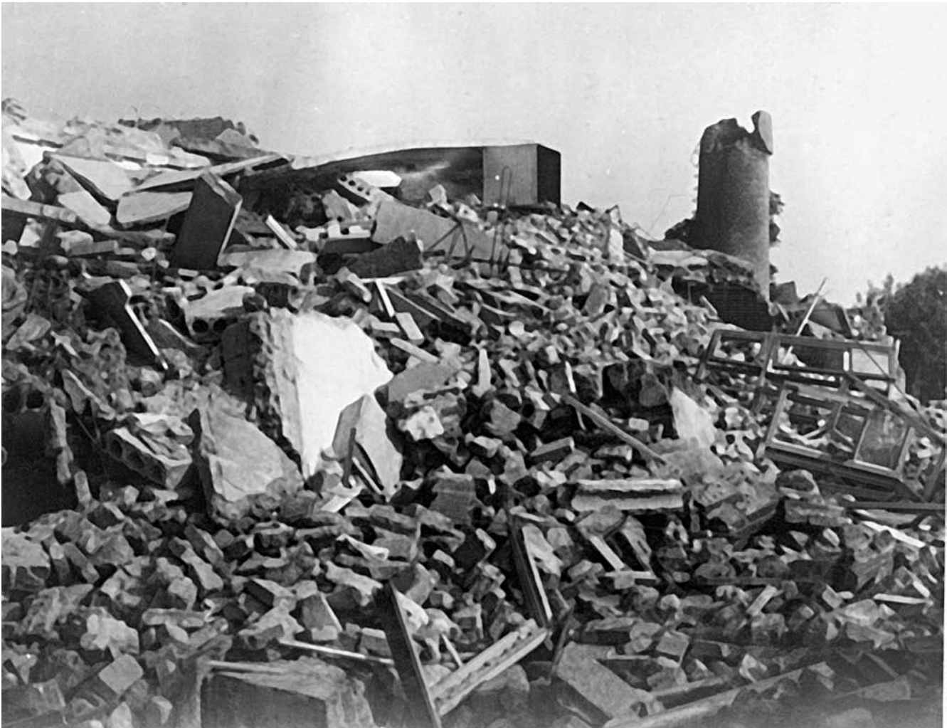
This four-story concrete and brick building of the Tangshan People's Bank completely collapsed into a pile of rubble during the 1976 Tangshan, China, earthquake. (Courtesy of the USGS)
