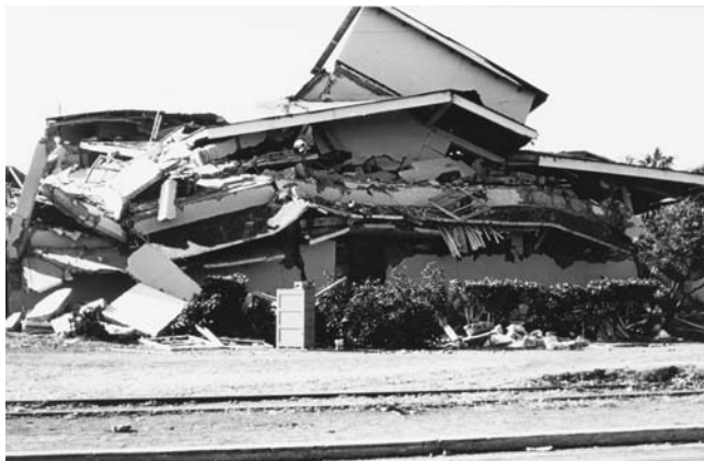
The 1972 Managua earthquake caused the collapse and complete destruction of this three-story, reinforced concrete Customs House office building. (Courtesy of the USGS)
