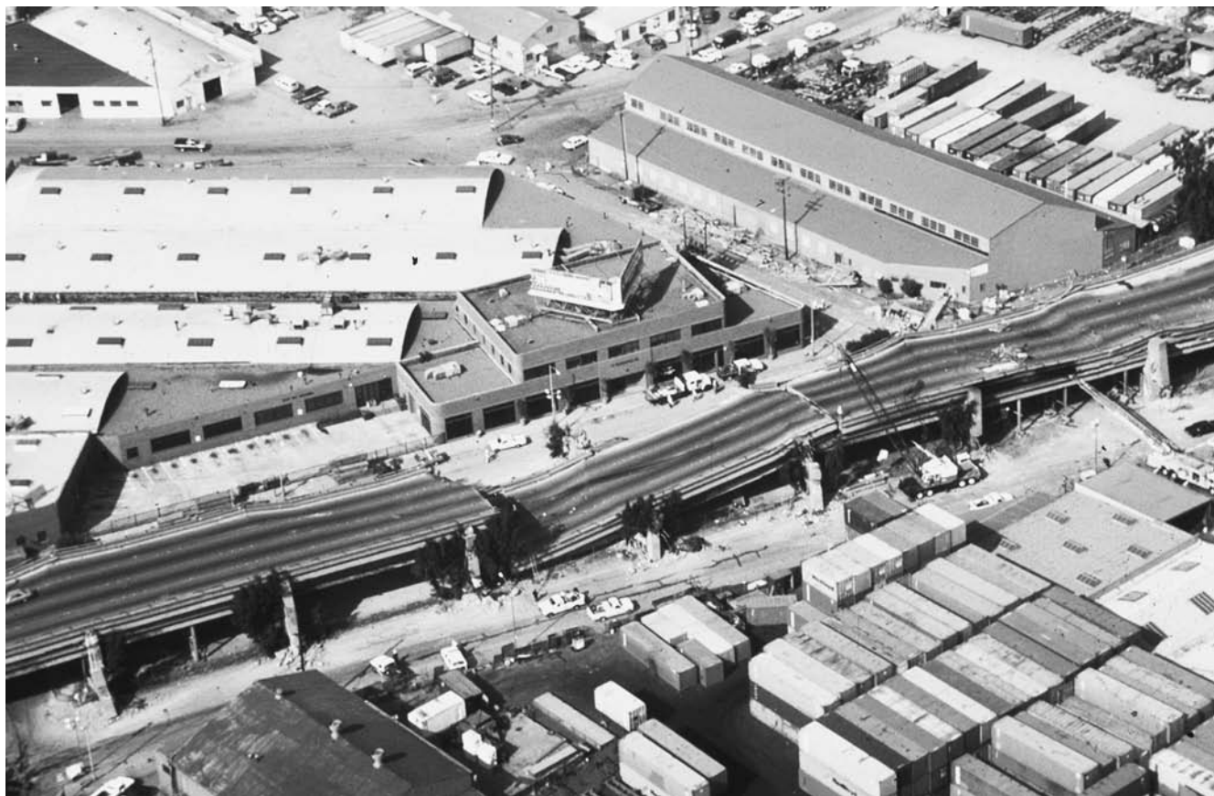
Aerial photograph of the collapsed Cypress viaduct of route I-880 in Oakland, California, as a result of the 1989 Loma Prieta earthquake. This collapse caused most of the casualties suffered during this event. (Courtesy of the USGS)
