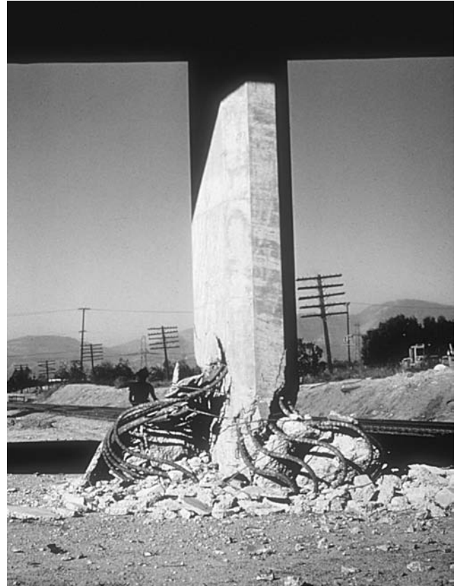
Crushing of the base of a column in an overpass during the 1971 San Fernando earthquake. The damage done to the column is characteristic of that done by a Rayleigh wave. The motion of the ground is like an ocean wave. The return upward motion causes the crushing because it is held in place by the overpass. (Courtesy of the USGS)
