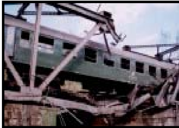
Figure 7-24. Example of a damaged rail transportation system.
