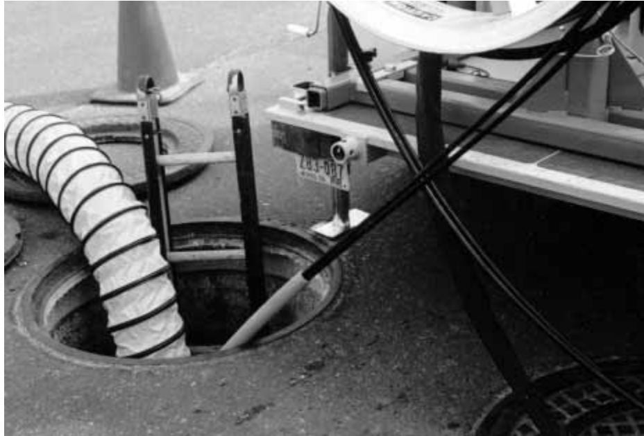
Figure 7-7 Two fiber optic cables being pulled through innerduct that has previously been pulled into conduit. Courtesy Condux
