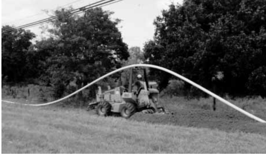
Figure 15-1 Fiber optic cable is often installed in conduit for outside plant applications.
