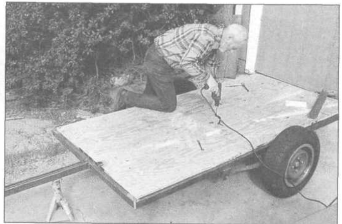
9.26 Locate where your tubes are and drill through the flooring and tubing, then bolt the floor down with carriage bolts, with the round heads on top so the floor is relatively smooth and a furniture dolly will go over the floor easily.
