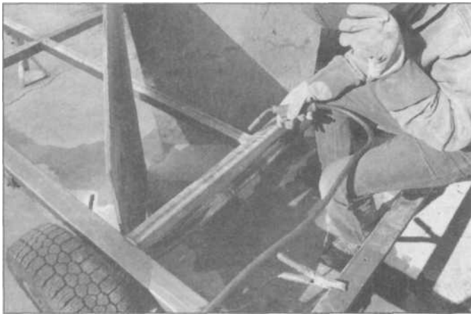
5.32 Gas-shielded MIGs are not made for outdoor work, but as long as you can keep the wind currents away, they work fine. On this driveway utility-trailer project, pieces of plywood are used as wind shields while welding.
