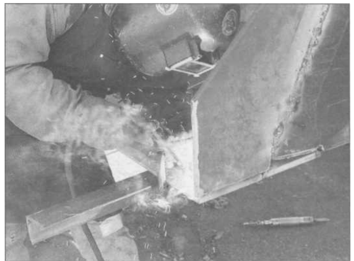
4.1 Arc welding will always be with us, as the best welding method for joining heavy plates for commercial, farm and industrial work. The weldor requires considerable protection from the spatter and radiation, usually wearing heavy leather protective gear.
