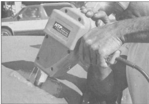
8.35 On a dented area that has been ground to clean metal, the tool is pushed in contact with the metal and the trigger is pulled for a half-second.
