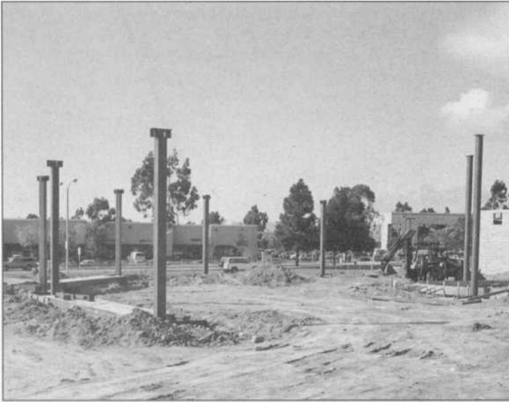
1.5 Wherever you see buildings go up, the basis for them is always steel, whether they wind up with wood, bricks or cement on the outside , it all began with the work of ironworkers and weldors.
