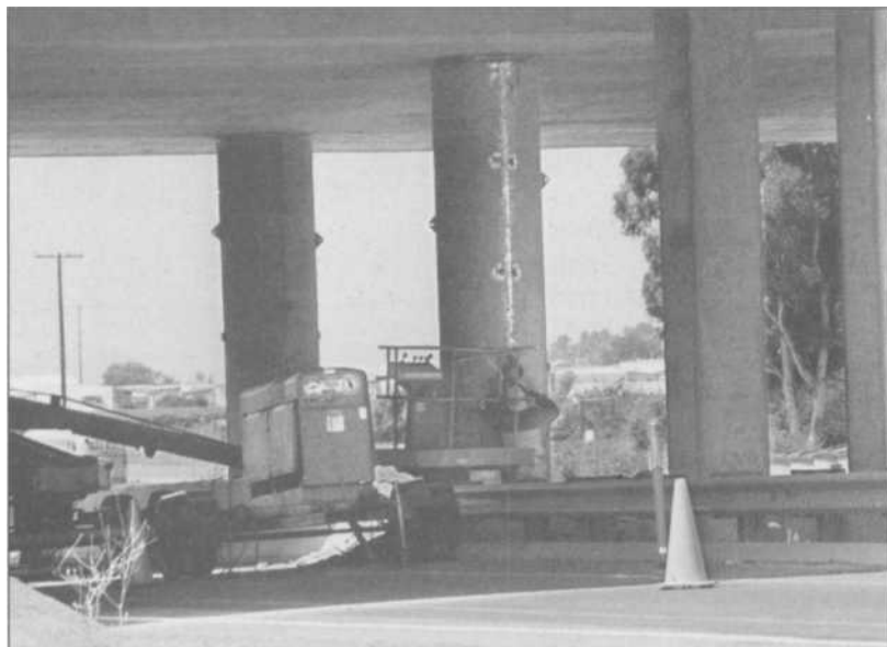
1.4 Under the center bridge column here are a welder (a machine) and a welder (a person). He is welding up steel enclosures for the concrete columns, to retrofit more strength in California bridges to meet newer earthquake codes.
