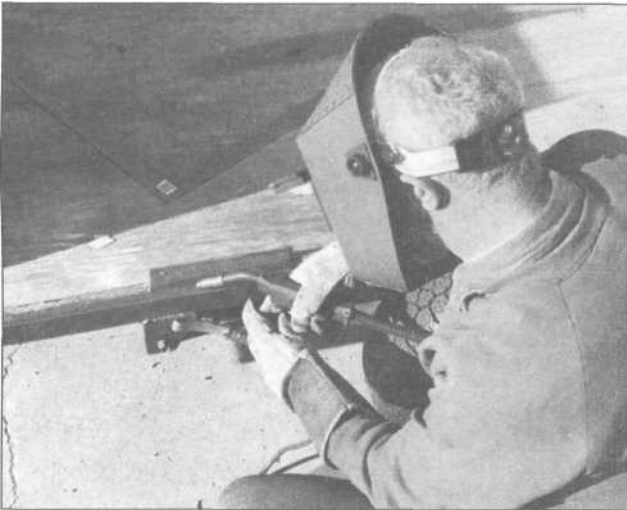
9.30 Short strips of 1/8-inch thick, 2-inch-wide strap metal (pre-drilled) were welded along the floor edges to help attach the bottom of the side panels. When MIG welding outdoors with argon gas shielding, use pieces of plywood around you to form a wind barrier to keep the gas from blowing away as you weld.
