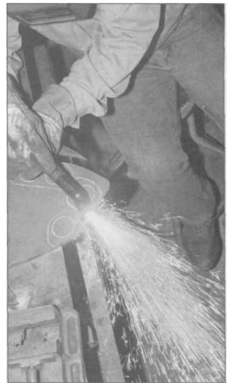
7.26 The 50-amp plasma cutter makes short work of cutting out the patterns and can easily pierce the center of a pattern to cut out internal holes and shapes.
