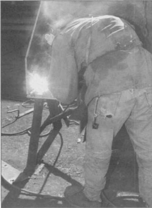
4.15 The arc spatter and radiation are dangerous. Do not allow any bystanders to observe the arc while you are welding. Also, notice how much smoke is around the weldor's helmet here. The fumes are dangerous and you should have an electric fan of some kind to blow it away from you when you are welding in a corner like this.
