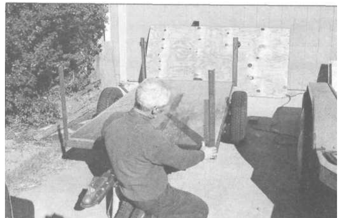
9.27 Four posts of heavy 1x2-inch angle-iron were welded on, one in each corner, as supports for the plywood sides. After welding, all were checked with a square.
