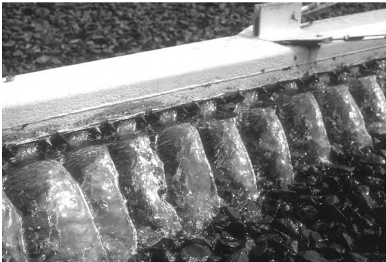
Figure 16.7 Attached growth wastewater treatment distributor.
