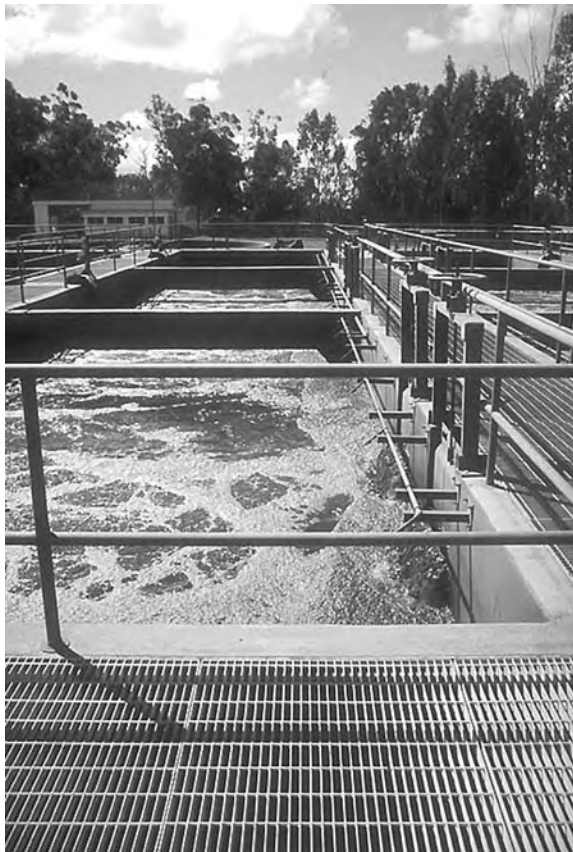
Figure 16.18 Suspended-growth (i.e., activated sludge) wastewater treatment facility.
