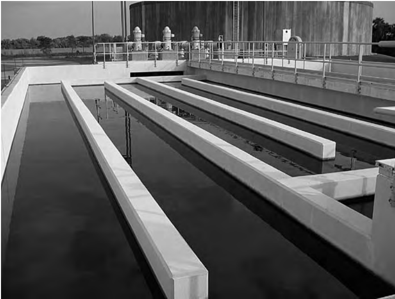
Figure 16.53 Serpentine chlorination reactor for wastewater effluent disinfection.
