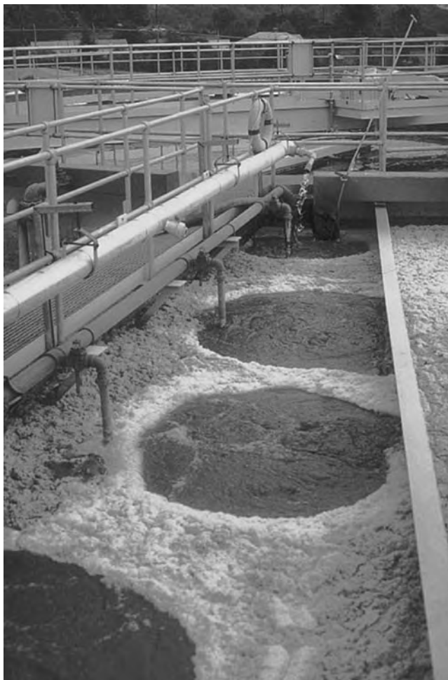
Figure 16.47 Aerobic sludge digestion system.
