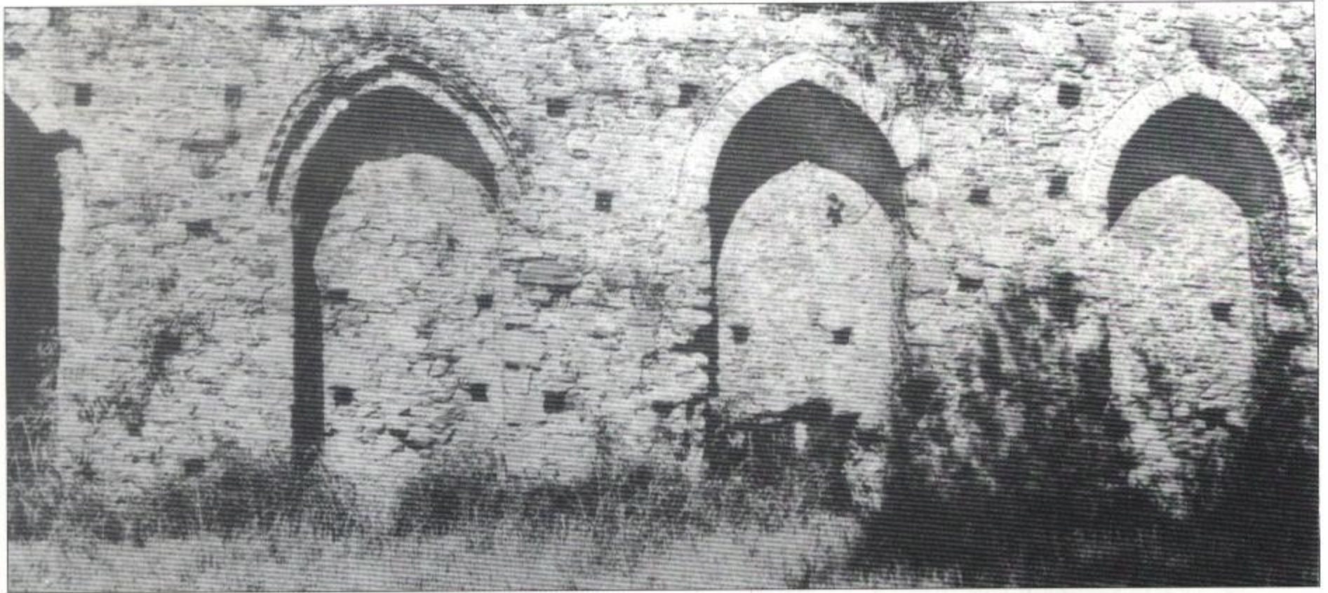
Interior of the north wall of the Crusader castle of Androusa, Greece. (Photograph A. Bon)
