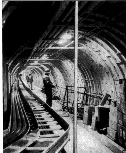
ABOVE: Work on the main tunnel of Titan I complex at Vandenberg AFB nears completion in 1960. Located 40ft. underground, the tunnel connected the launch center to the missile launch silos. (National Air and Space Museum, Smithsonian Institution)
