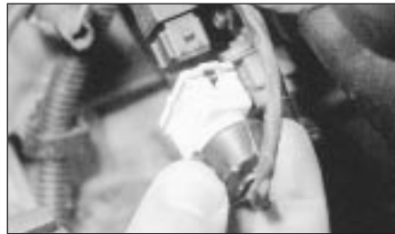
B The throttle potentiometer wiring plug may cause problems if not connected securely.
