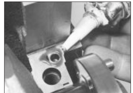
18.71 Applying sealant to the cylinder block No 1 main bearing cap mating face
