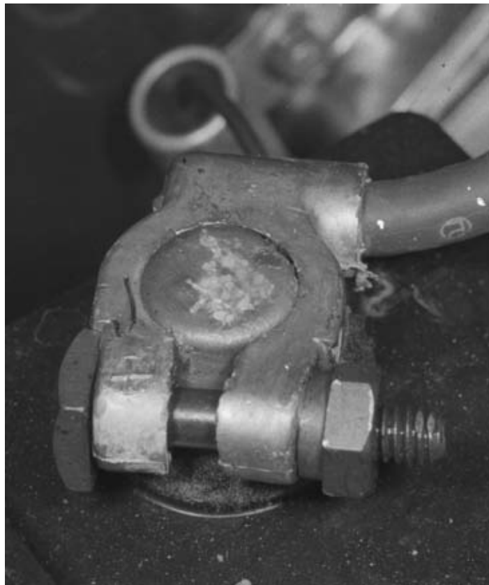
Figure 7-11. The most common type of top terminal battery clamp.
