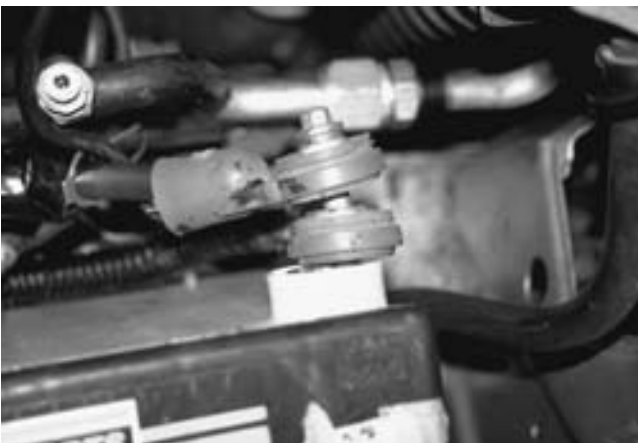
FIGURE 15-11 Carefully inspect all battery terminals for corrosion. This vehicle uses two positive battery cables connected at the battery using a long bolt. This is a common source of corrosion that can cause a starting (cranking) problem.
