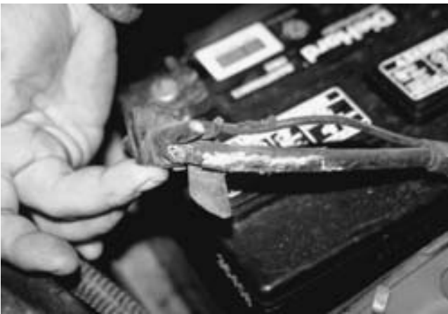
FIGURE 15-10 This battery cable was found to be corroded underneath. The corrosion had eaten through the insulation yet was not noticeable until it was carefully inspected. This cable should be replaced.
