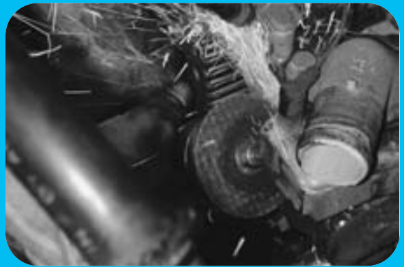
STEP 16 To save time, this service technician is cutting off the head of one bolt that holds a support bracket. This bolt cannot be removed without removing the entire intake manifold.
