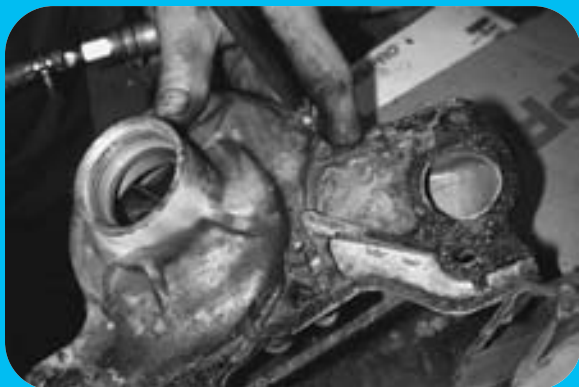
STEP 21 The replaceable part of the water pump has to be removed from the housing. There is a hidden Phillips screw on the backside that has to be removed.
