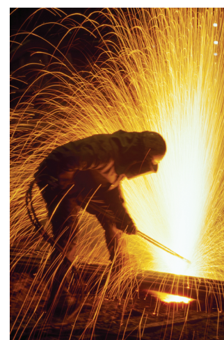
FIG. 5.12 Cutting steel with an oxyacetylene torch. An oxygen–acetylene flame is used to heat steel until its glowing red hot. Then the acetylene is turned off and the steel is cut by a stream of pure oxygen whose reaction with the hot metal produces enough heat to melt the steel and send a shower of burning steel sparks flying. (Scott T. Smith/Corbis Images.)
