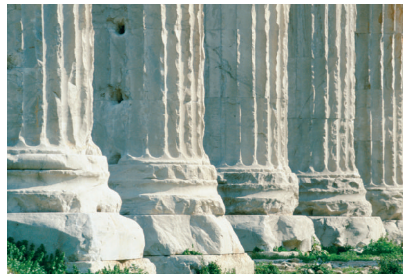
FIGURE 6.2 Even the most “solid” monuments that people erect eventually yield to the day in and day out attack of weathering processes. Temple of Olympian Zeus, Athens, Greece. (Photo by CORBIS)
