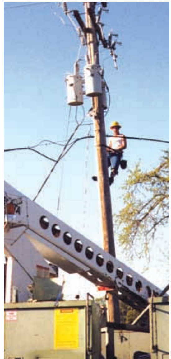
▲ A sign of the times. Like electricity and gas, cable television also has to be restored as soon as possible.
