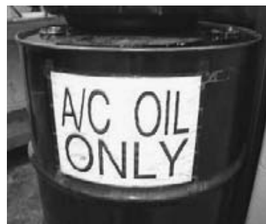
FIGURE 2-8 Used refrigerant oil should be stored in a clearly labeled, secure container. (Courtesy of James Halderman)
