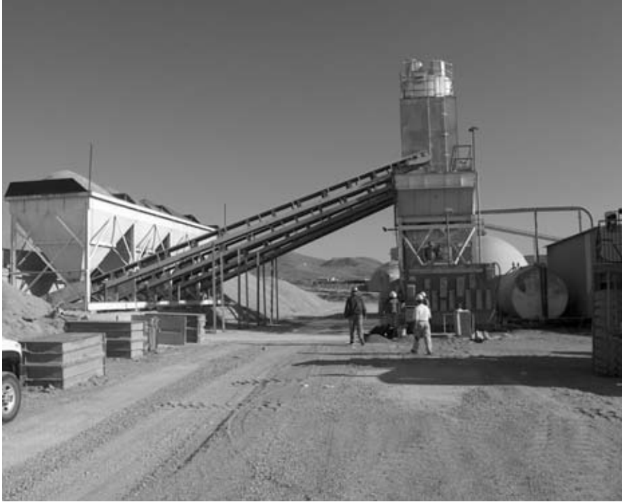
FIGURE 7.4 Concrete ready mix plant.
