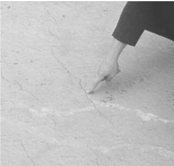
FIGURE 7.27 Plastic shrinkage cracking.
