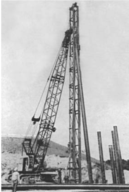
FIGURE 10–26 Pile installation. Source: Courtesy of Associated Pile & Fitting Corporation of New Jersey.
