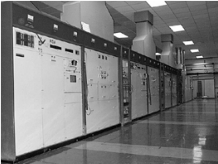
Figure 2.4 High power Medium Wave transmitters at Brookmans Park transmitting station (Courtesy Crown Castle International)
