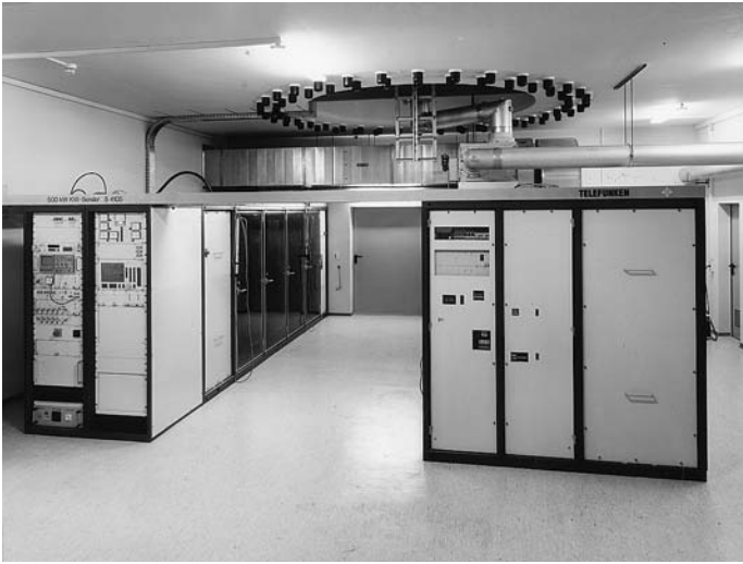
Figure 2.2 Telefunken transmitter (Courtesy Telefunken Sendertechnik GmbH)
