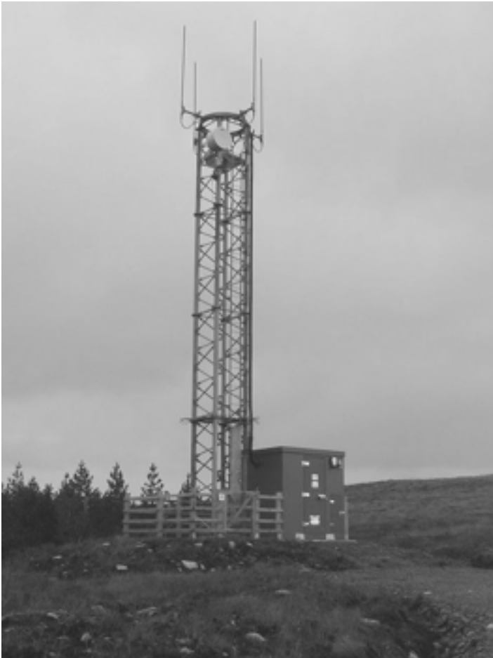
Figure 6.13 Tower mounted colinear antennas (Courtesy of BT)
