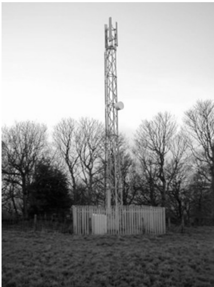
Figure 6.12 Tower-mounted sectored antennas (Courtesy of BT)
