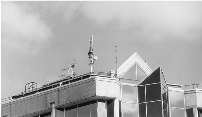
Figure 6.20 Roof mounted equipment – glass and brick structure (Courtesy of E. Randall)
