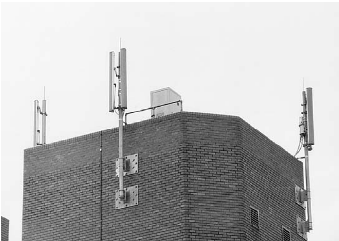
Figure 6.19 Roof mounted equipment – Brick building (Courtesy E. Randall)
