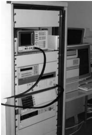
Figure 7.2 A relatively simple anechoic antenna range instrumentation setup showing a microwave synthesizer, an IEEE-488-type switch matrix, and a high-end spectrum analyzer.
