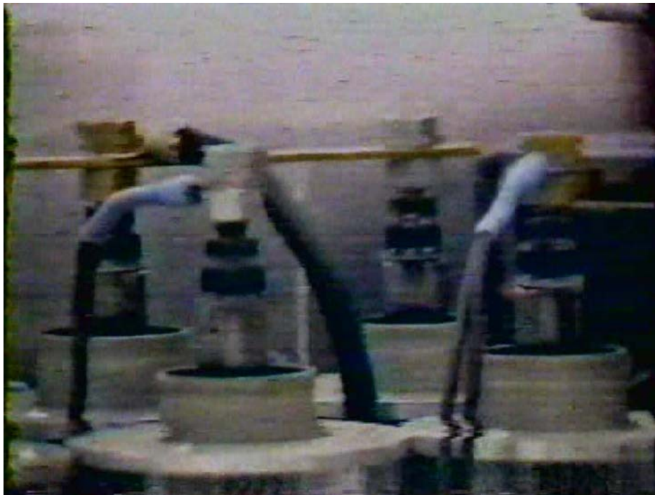
Ignitrons installed on the “Red Motor Cart”
