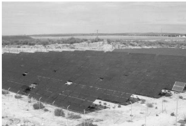
Figure 22.1 The 1 MWp ground-mounted system in Toledo, Spain. Reproduced with permission by BEAR Architekten T. Reijenga
