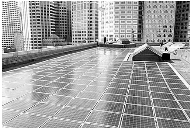
Figure 22.8 Powerguard flat-roof PV system including thermal insulation at the Coastguard building in Boston, MA (USA). The 3 kWp system has a special wind-tunnel-tested profile at the edge to keep the system on the roof in heavy winds. Adapted from Eiffert P, Kiss G, Building-Integrated Photovoltaic Designs for Commercial and Institutional Structures – A Sourcebook for Architects , 42–44, NREL, Golden, CO (2000). Reproduced with permission by NREL USA [18]
