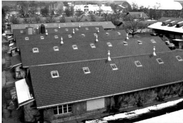
Figure 22.15 The 80.5 kWp Atlantis Sunslates on the roof of the historic horse stables in Bern (CH). The color and texture matches so well that this PV system was allowed on a protected historic building. Reproduced with permission by Atlantis Solar Systems Ltd
