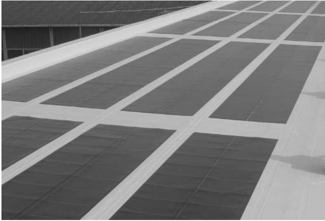
Figure 22.36 Alwitra Evalon® roofing foil with amorphous silicon cells. Reproduced with permission by O.Ö. Energiesparverband
