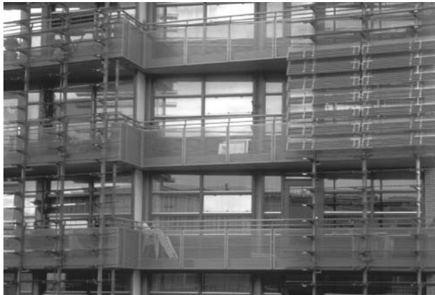
Figure 22.41 ADO louver system with integrated transparent PV modules at an apartment building in Amersfoort Nieuwland (NL). The automatic louvers can switch in two positions. The horizontal position at night (left on the figure) and tilted to the sun by day (right on the figure). Reproduced with permission by BEAR Architecten T. Reijenga
