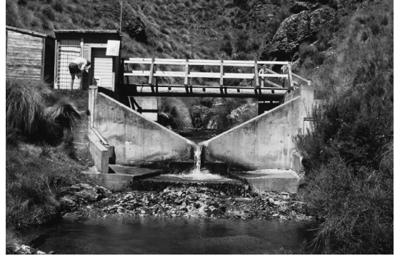
Figure 5.11 A V-notch weir. The water level in the pond behind the weir is recorded continuously.
