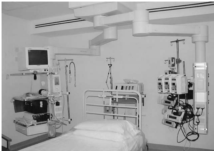
FIGURE 12 Burn ICU beds should be spacious and should have independent thermostats to permit changes in room environmental conditions according to patient needs.
