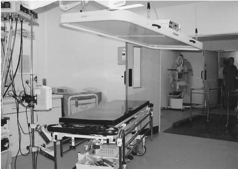
FIGURE 11 Thermal panels or heat radiators provide a central area of high temperature over the patient, allowing a lower temperature in the rest of the environment for staff and visitor comfort.
