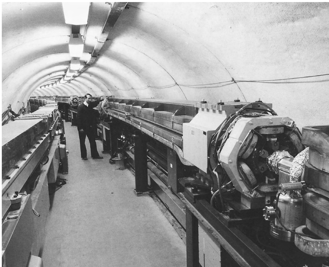
View inside the tunnel for CESR. The booster synchrotron is on the left, the storage ring on the right. CREDIT: COURTESY OF CORNELL UNIVERSITY.
