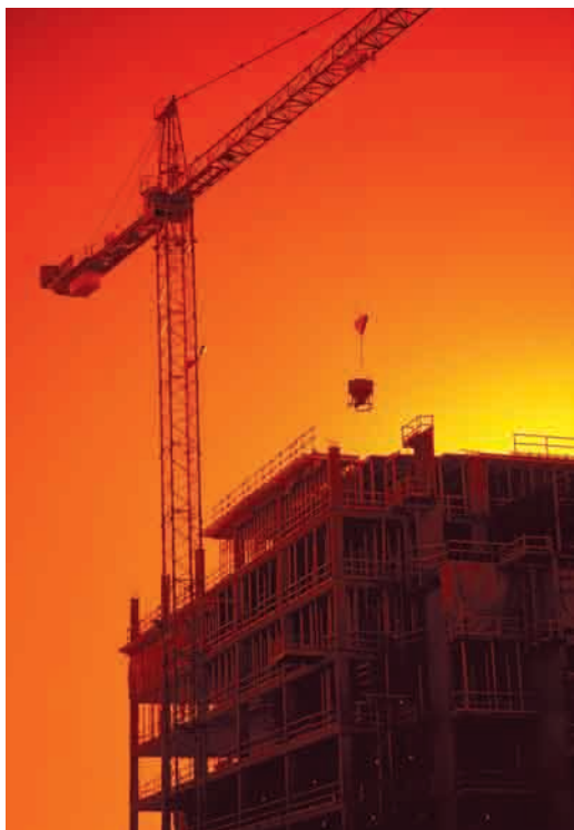
Figure 1.10 Mobile construction cranes can withstand the tension necessary to lift loads of up to 1000 t.
