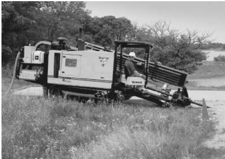
Figure 5.13. Directional boring machine in use. (Photo courtesy of Vermeer Manufacturing Company; www.vermeer.com .)
