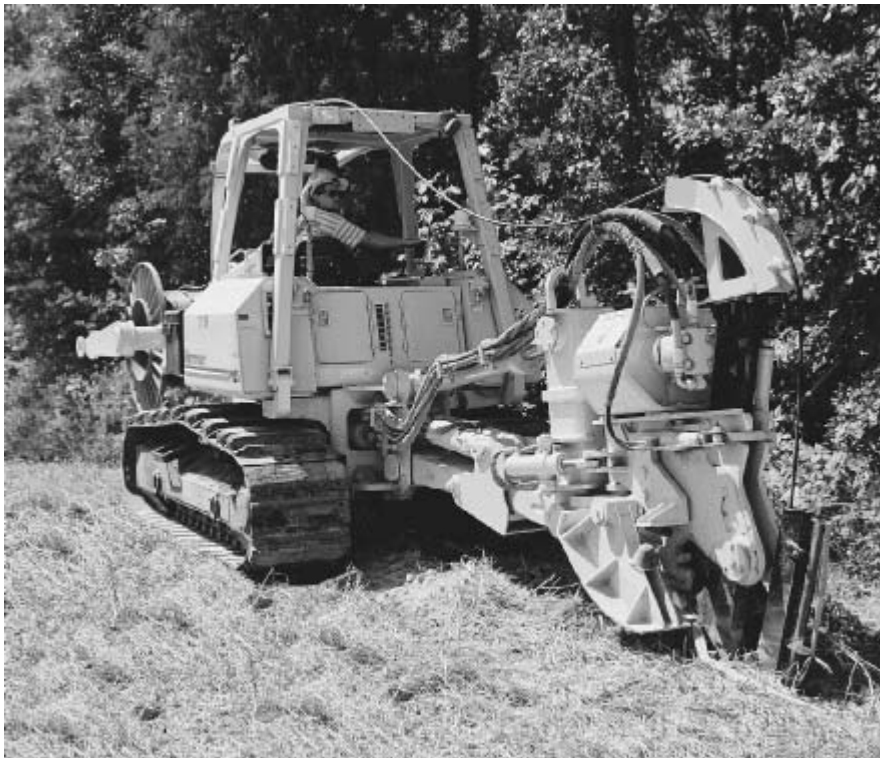
Figure 5.12. Plowing operation for direct burial of optical fiber cables. (Photo courtesy of Vermeer Manufacturing Company; www.vermeer.com .)
