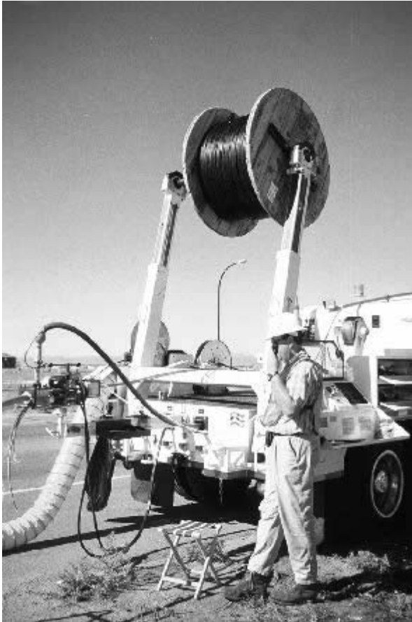
Figure 5.16. Microducts being fed into the mechanical drive of a cable jetting machine. (Photo courtesy of Sherman & Reilly, Inc.; www.sherman-reilly.com .)
