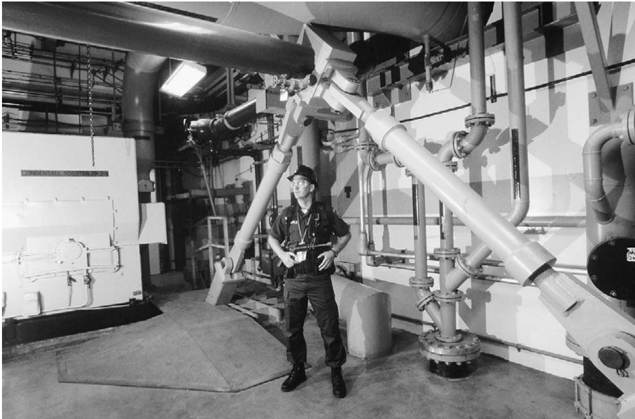
A security officer stands next to a seismic brace inside the Diablo Canyon Nuclear Power Plant. Braces like these are representative of the technological advances in earthquake engineering. (© Roger Ressmeyer/Corbis.)
