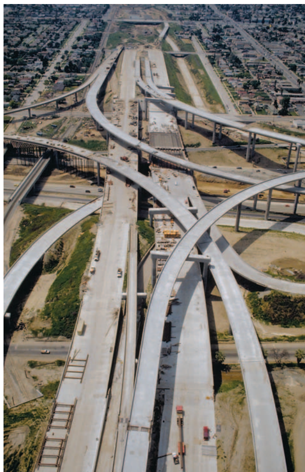
An aerial shot of a freeway system under construction in southern California. Photograph by Tom Carroll. Phototake NYC. Reproduced by permission.
