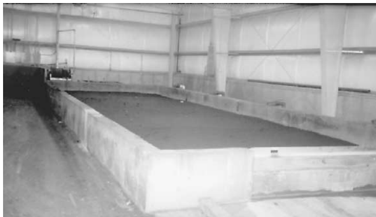
Figure 3.125 A vacuum-assisted drying bed.
