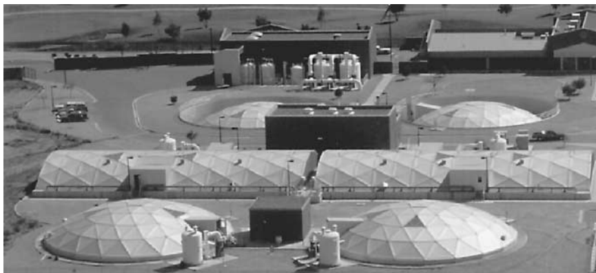
Figure 5.66 Photograph of a wastewater treatment plant with covered primary, secondary, and sludge-treatment operations. (Courtesy of CONSERVATEK, Inc.)
