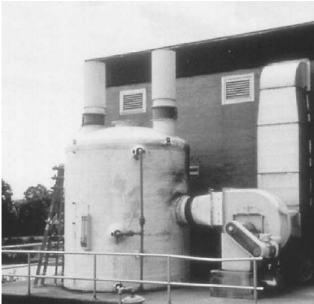
Figure 5.81 Photograph of an activated-carbon adsorption system. (Courtesy of Environmental Systems Division PURAFIL, Inc.)
