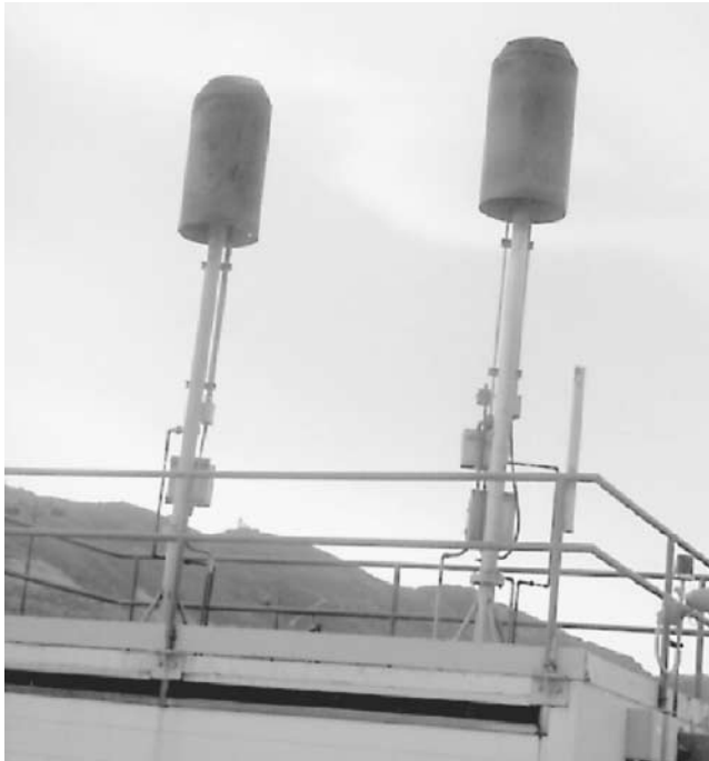
Figure 3.25 A flare system used to burn excess digester biogas.
