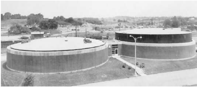
Figure 3.37 A two-stage anaerobic digester system. (Courtesy of Dorr Oliver.) (Note the additional gas storage capacity in the digester tank fitted with floating gas-holder cover.)
