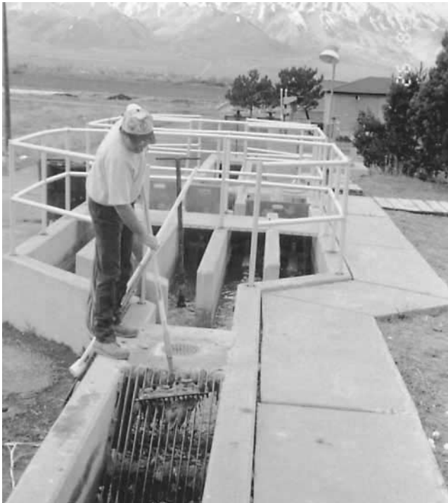
Figure 2.74 An operator manually cleaning a bar screen.
