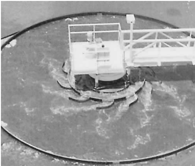
Figure 2.28 (a) Schematic diagram of primary sedimentation of wastewater designed for induced flocculation. (b) Primary clarifier equipped with an energy-dissipating inlet for enhanced flocculation. (Courtesy of WesTech Engineering, Inc.)
