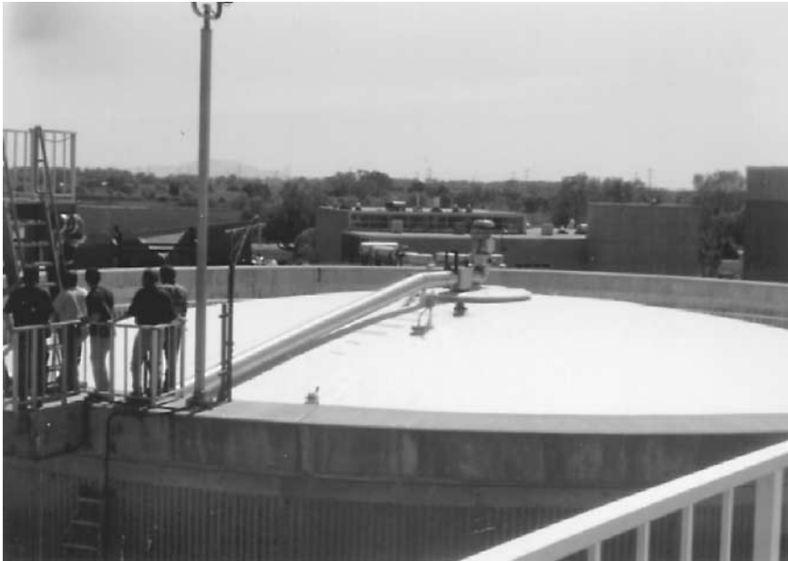
Figure 5.35 An anaerobic digester equipped with a floating cover.
