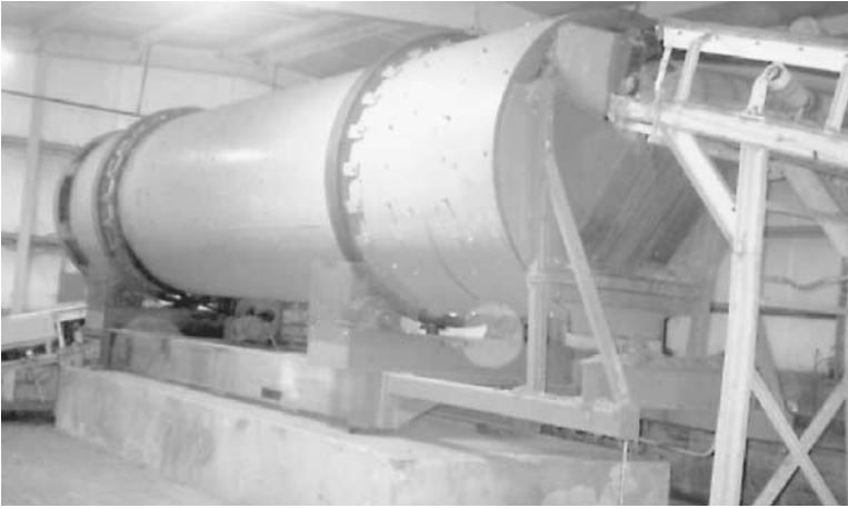
Figure 3.77 Rotational mixer used to prepare sludge–bulking agent mixtures.
