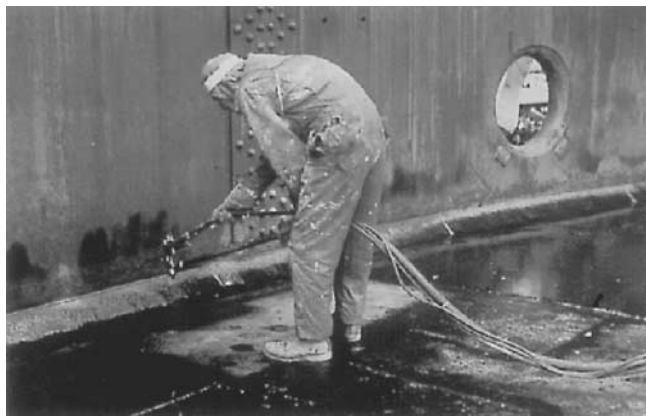
Figure 5.96 Photograph of coating applied to tanks for corrosion control. (Courtesy of C.I.M. Industries, Inc.)
