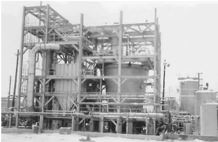
Figure 1.34 Full-scale hot windbox fluidized-bed incinerator system. (Courtesy of Infilco-Degremont, Inc.)
