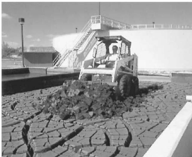
Figure 3.126 Photograph of “cracked” (i.e., dewatered) sludge being removed from a vacuum-assisted drying bed. (Courtesy of U.S. Environmental Products, Inc.)
