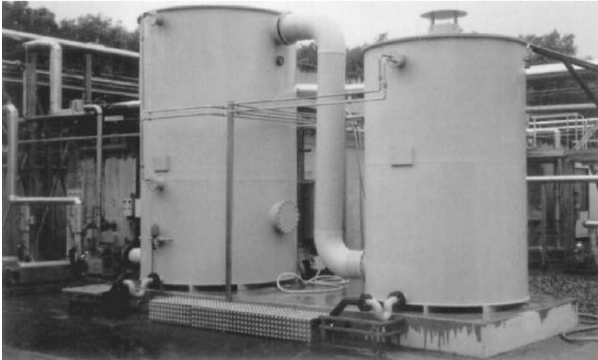
Figure 5.93 Photograph of a two-stage bioscrubber system. (Courtesy of BIOWAY.)
