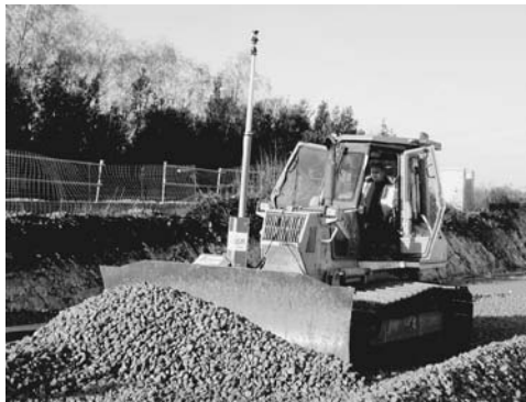
Figure 12.30 Use of GPS satellites for mapping and construction (Reproduced by permission of © Leica Geosystems)
