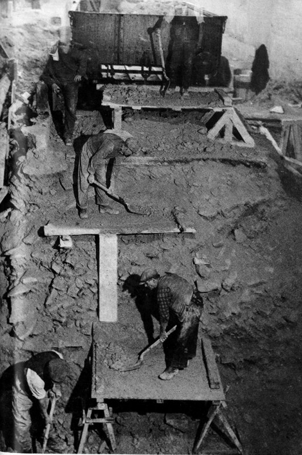
31. Deep excavation under way in the station area of Tunnel Quarry during 1936. Waste is thrown up from platform to platform to be loaded into the GWR 10-ton open truck parked at the end of the original underground siding.
