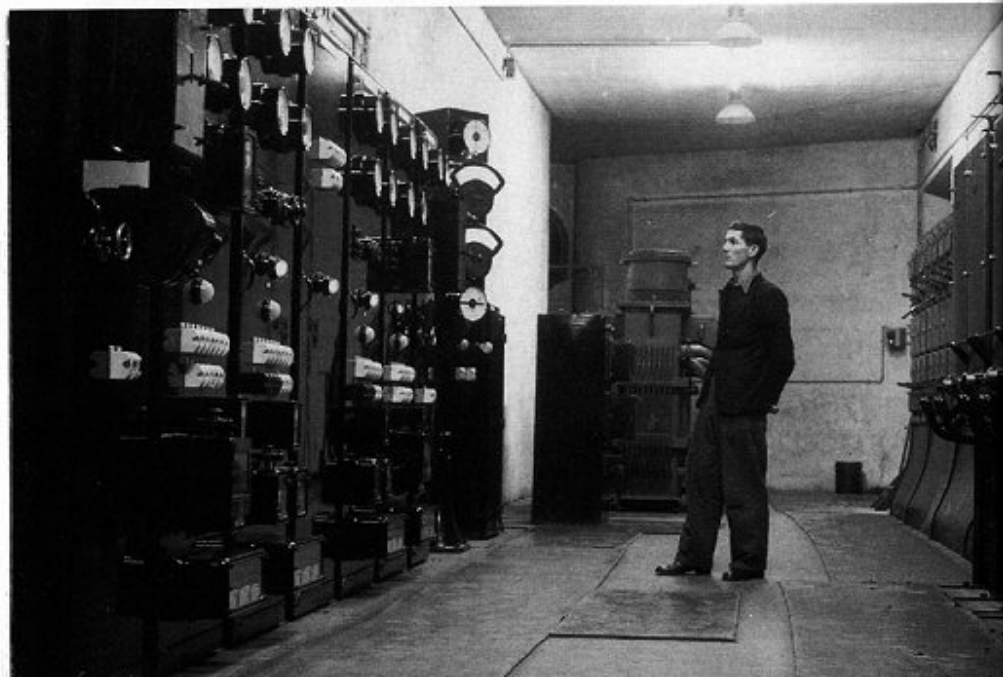
8. Tunnel Quarry switchroom, with transformers in the background and indicator panels on the left.
