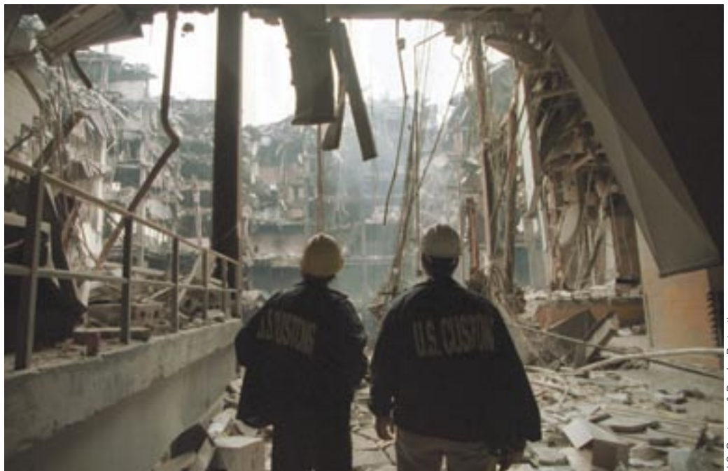
Surveying the wreckage: Customs agents review the damage from inside the NYC Customhouse after the terrorist attack.
