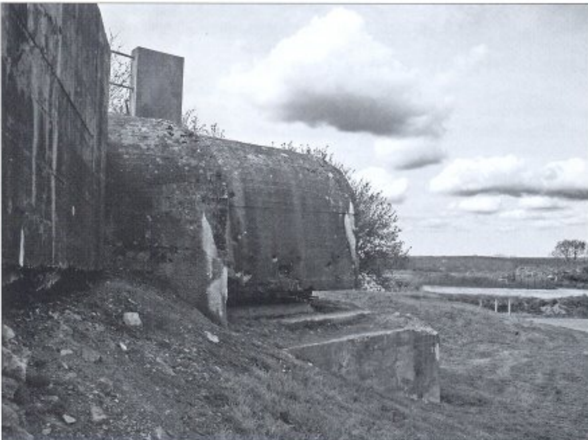
A view of the observation post of MKB St. Marcouf today with the wartime damage repaired. This was an SK design peculiar to the site and not a standard design. (Author's collection)
