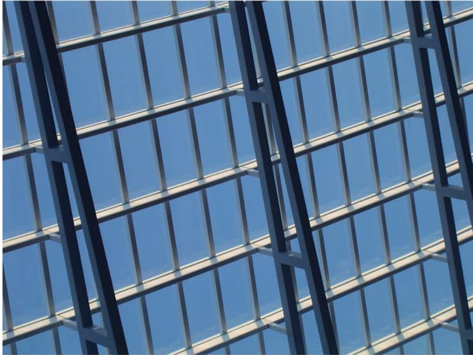
Steel Network Across the Firmament A transparent part of the New Academic Complex's roof reveals the grid used for support
