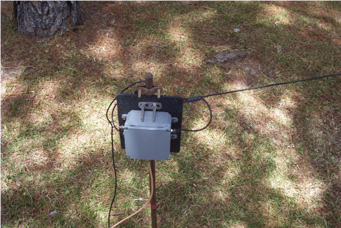
Feed Point of AS-WV-xxx Antenna showing balun mounted to plate and attached to antenna wire.
