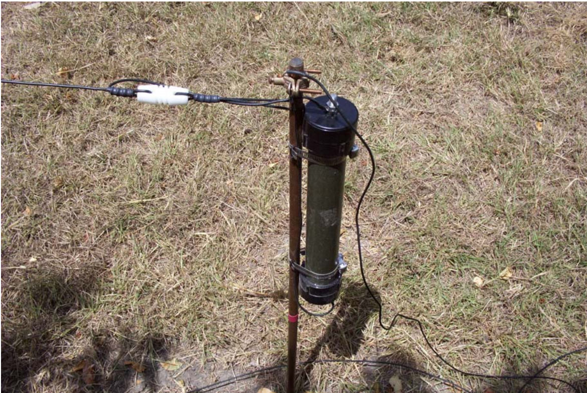
Termination detail of AS-WV-XXX Antenna, showing strain relief insulator system, Rugged Load, and ground rod.
