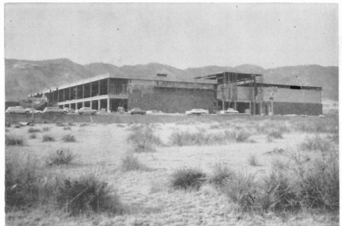
Two recent fires at construction site of new Colorado Springs plant are not expected to delay completion this summer.
