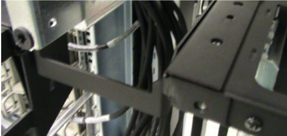
Figure 4-7 Rack Bonding Spacer – Top of Rack
